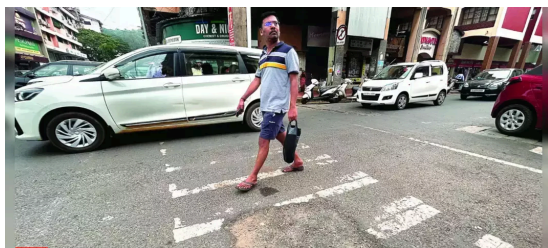
Faded Pedestrian Crossing
