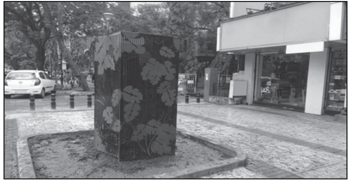
Photo 11 Covered and Painted Electrical Feeder Pillar Boxes
