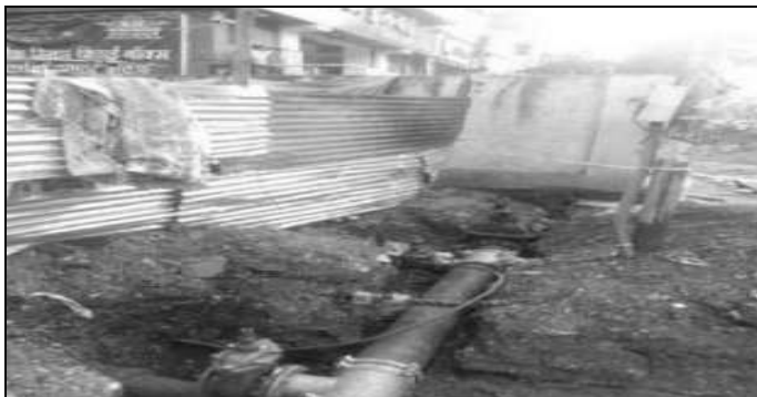
Photo 43 Individual Property Connections from Main Water Line
