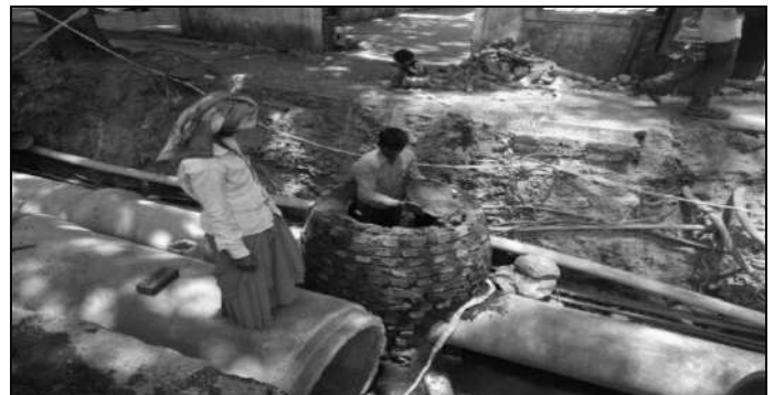
Photo 44 Individual Property Connections from Main Sewer Line
