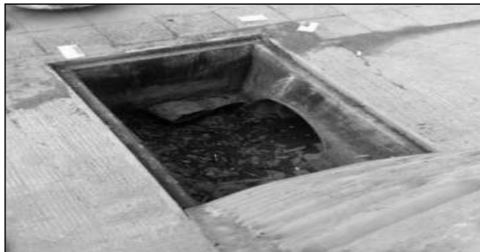
Photo 46 Individual Property Connections to Main SWD Line Chamber
